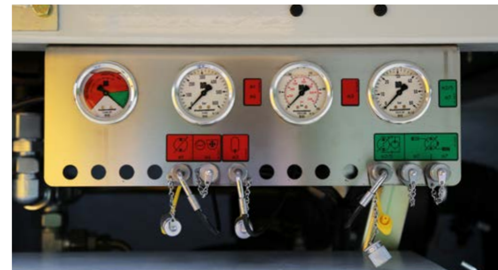
Mini-measuring strip: All hydraulic measuring points at a central location (BSA latest generation)
