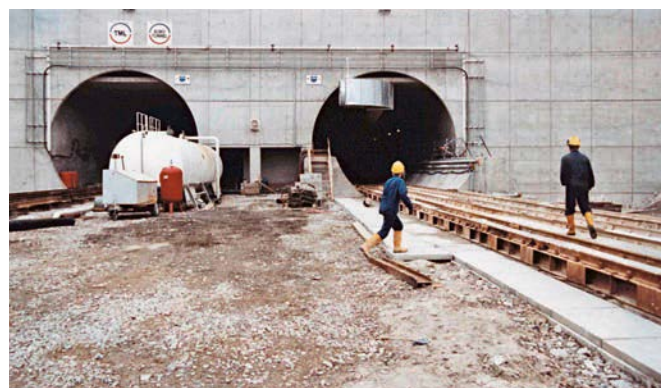
THE BIG BREAKTHROUGH Since 1st December 1990, the tunnel has connected Great Britain with the European continent under the sea bed. 15,000 workers worked on it for three years, seven days a week.
