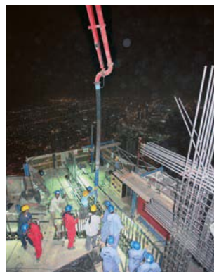
IN THE COOL OF THE NIGHT In Dubai, the work was mainly carried out at night, as there was the risk of it hardening prematurely due to the high daytime temperatures.
