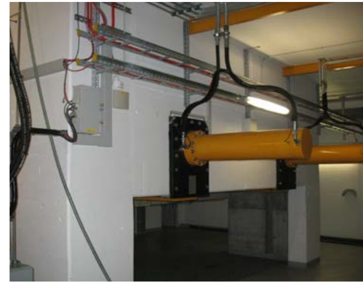
Sliding frame cylinder in a concrete silo, Sewage sludge plant Oftringen, Switzerland
