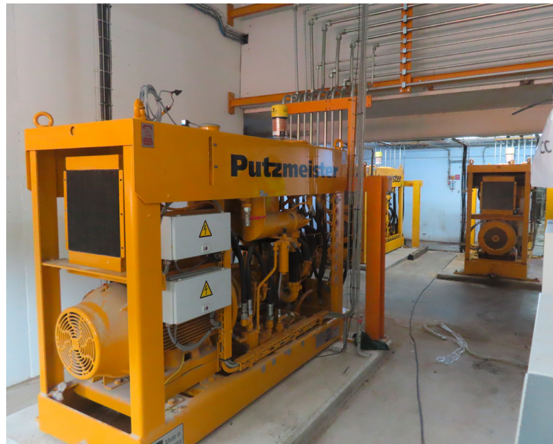
HA 55 E hydraulic power pack of the third line, the other two are visible in the background
