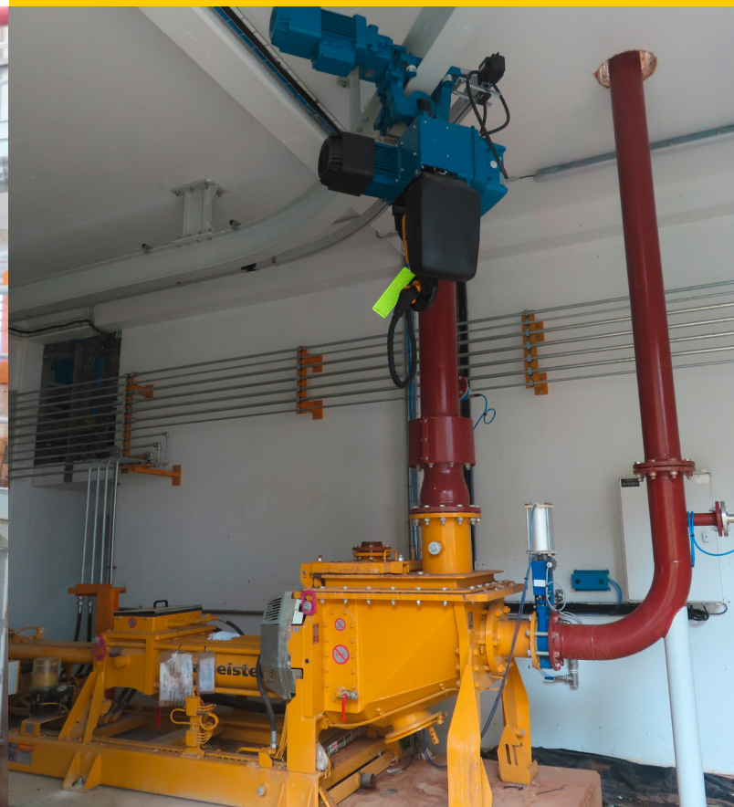
Third recirculation pump
