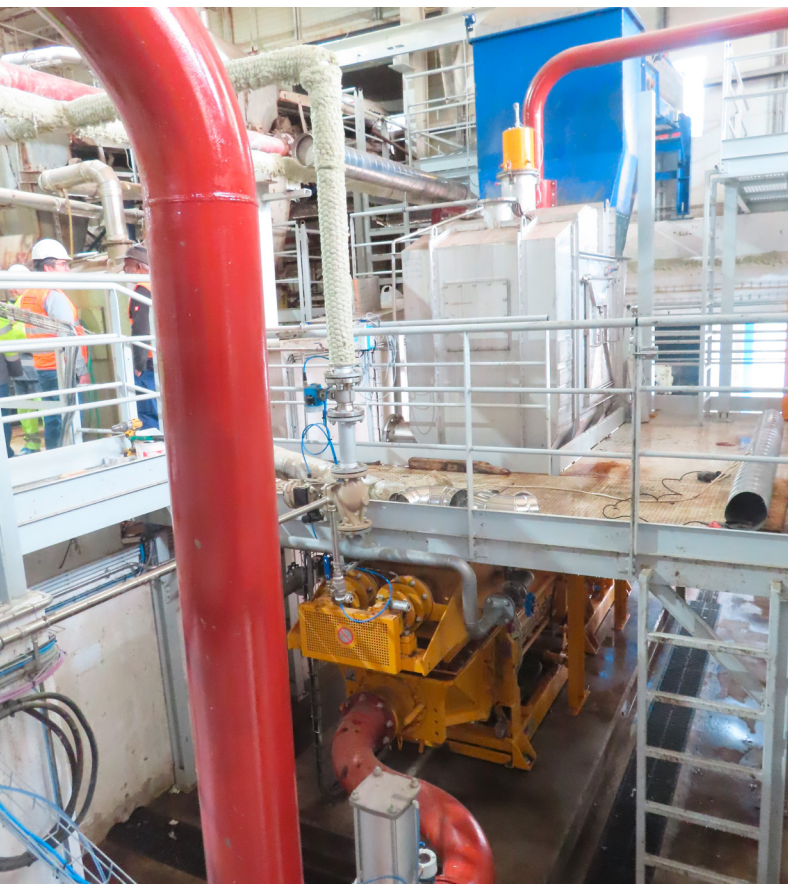
Reception hopper, screw conveyor and feed pump of the third line. You can also see how the recirculation pipework returns to the reception hopper
