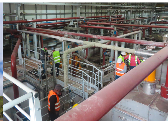
View of the plant
