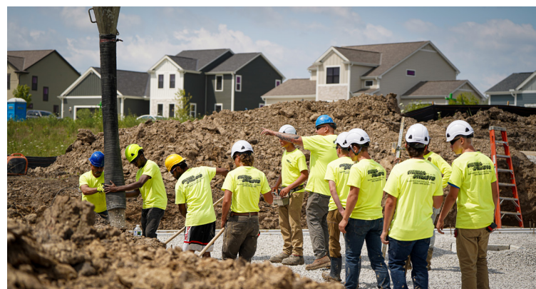
One student runs the Putzmeister Telebelt® 110 while another ensures the concrete is poured properly under supervision from Perma-Structo employees
